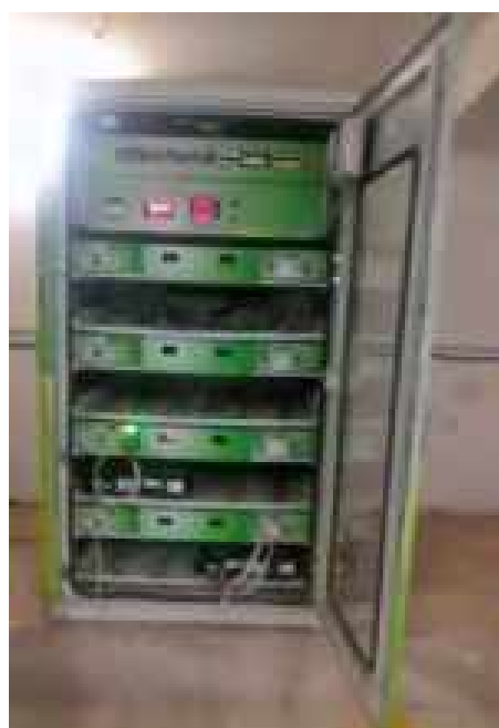
FIGURE 25: BULK BATTERY CHARGER USED BY OLA ELECTRIC IN NAGPUR
