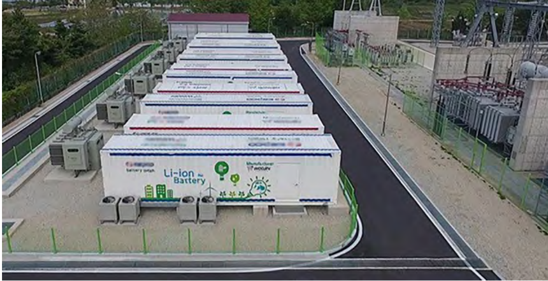
Figure D.4: Sokcho Battery Energy Storage System
